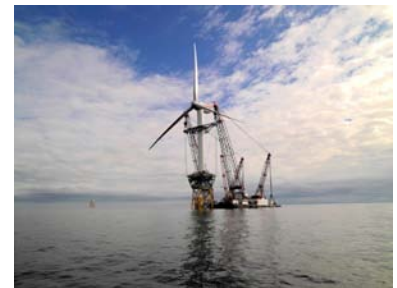
Figure 10.8. Construction of the Beatrice demonstrator deep offshore windfarm. Photos kindly provided by Talisman Energy (UK) Limited.
